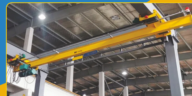
UNDER SLUG EOT CRANE
