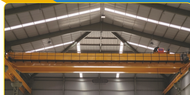
DOUBLE GIRDER EOT CRANE
